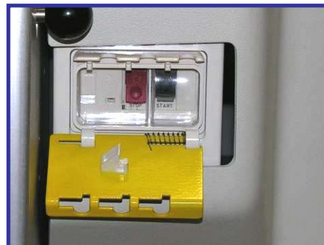
Main Power Switch
